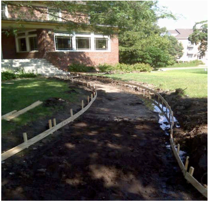
The existing bush and light pole at the intersection of the old sidewalk and parking sidewalk was removed as a part of the sidewalk renovation project. This is a view from the chapter house to the street.
